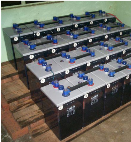
Photo 1: Wet lead acid batteries 2V/700Ah
