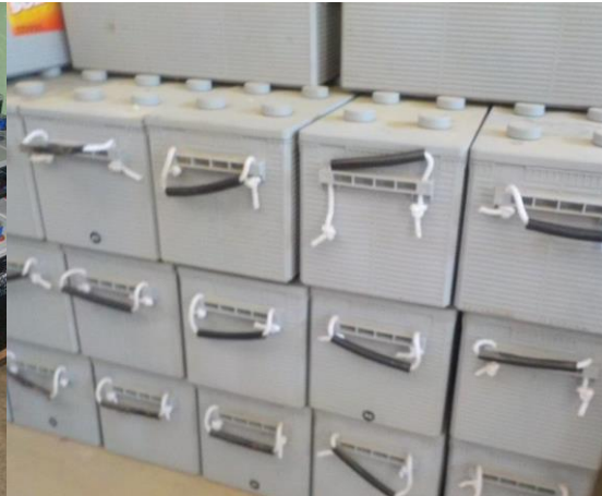
Photo 2: Aged free maintenance batteries 2V/210Ah at the health centre
