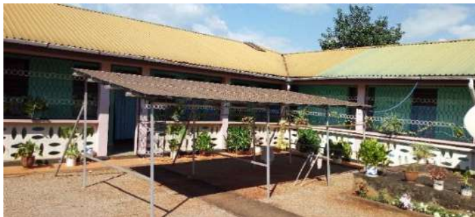
Photo 15: 2.96kWp solar system at St. Ann Sisters, Morogoro ©TAREA
