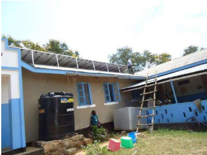
Photo 18: Solar photovoltaic system at Magubike Health Centre, Morogoro Region ©TAREA
