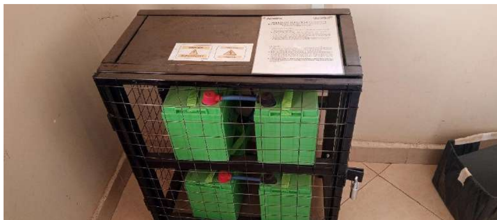
Photo 8: Battery Bank at Mutukula Dispensary
