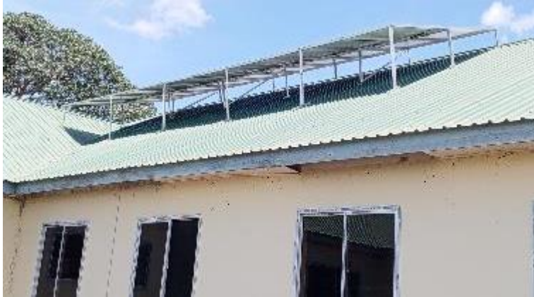
Photo 7: Solar panels for the school compound
