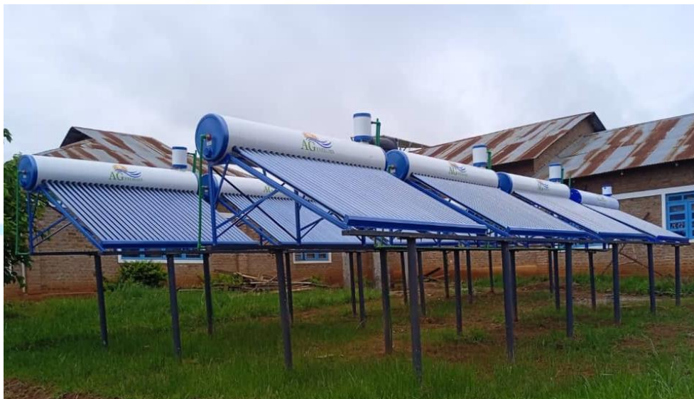
Photo 1: 2500 litres solar water heating plant at the Emmaberg Girls High School
