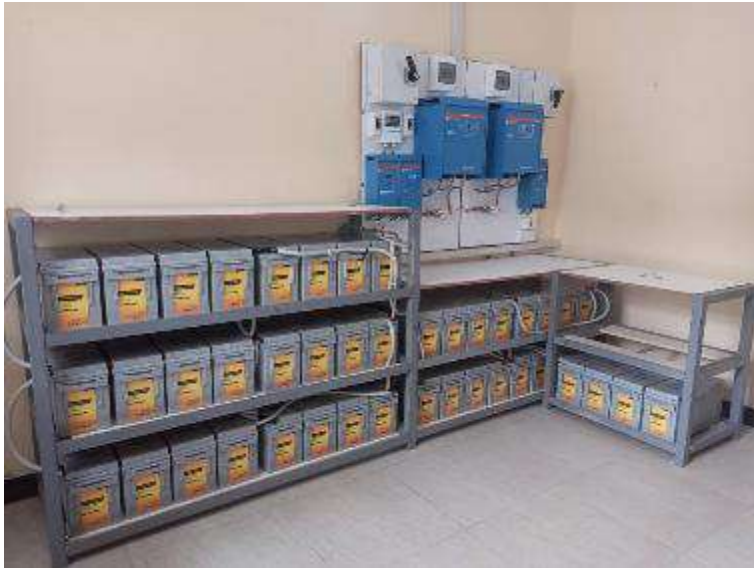
Photo 1: Solar energy storage at Chiungutwa Health Centre, Masasi
